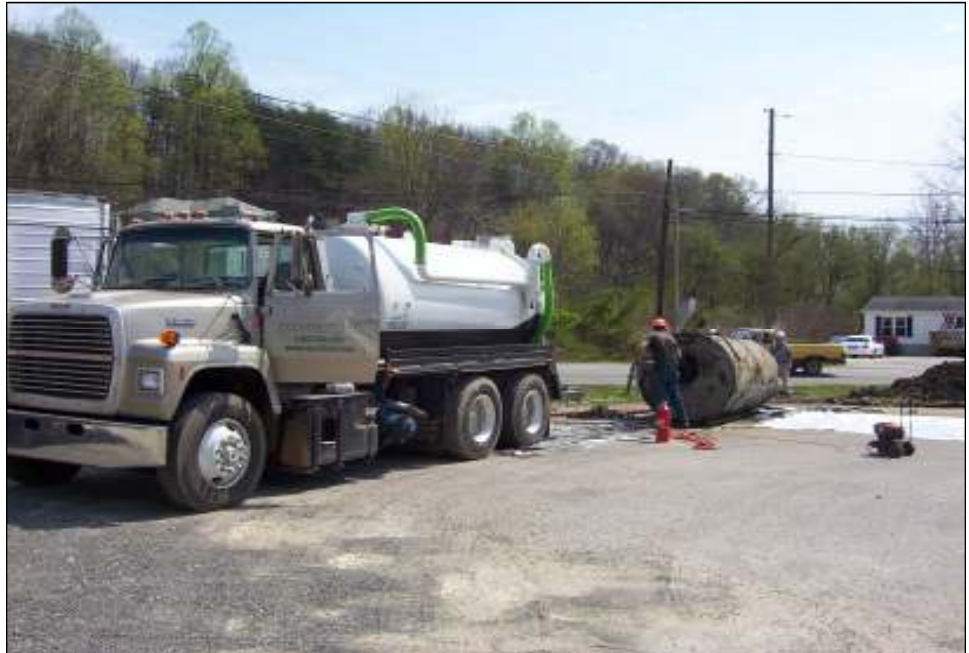
ECO-FIRST employee Sterling Ayers pressure cleans the interior of an underground storage tank during a Summer 2005 removal near Ashland, KY. Photo by ECO-FIRST, Inc.
