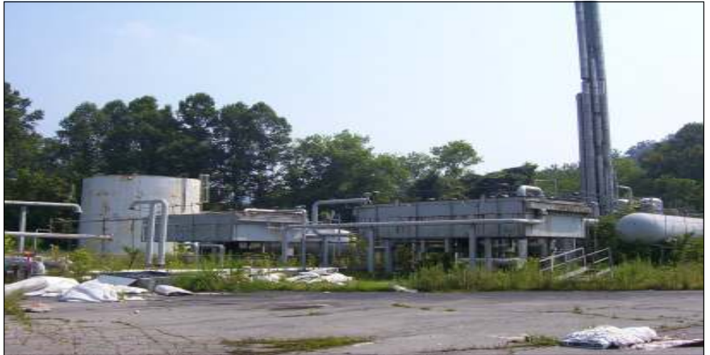
ECO-FIRST recently completed the demolition and recycling of this natural gas compressor station in Eastern Kentucky at no cost to the property owner/operator. Photo by ECO-FIRST, Inc.
